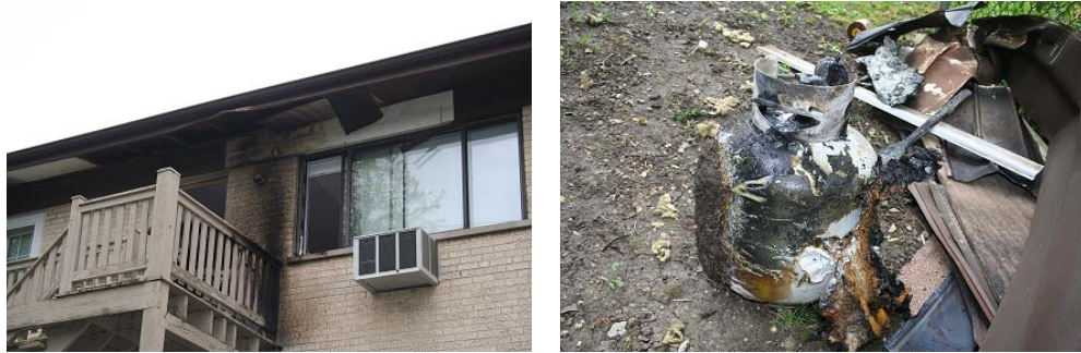
Damage resulting from the May 1 grill fire
